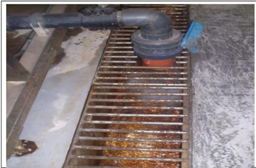
Figure 16 Reverse osmosis water rejects area
