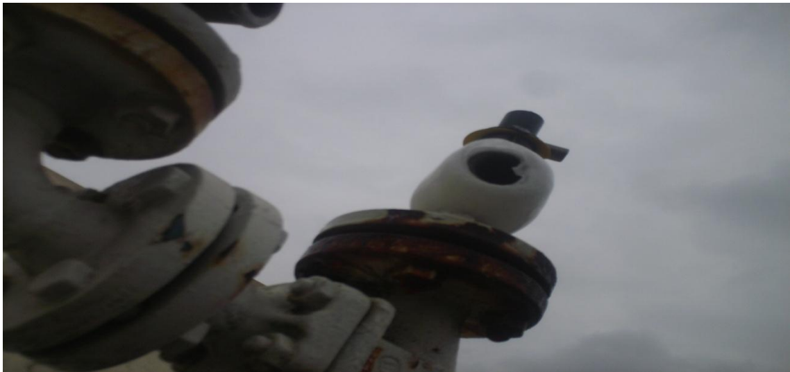
Figure 18 Leaking CO 2 safety valve
