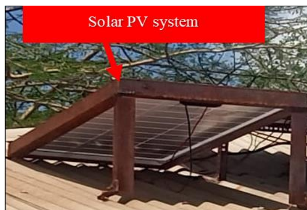
Plate 3.10: Solar PV System Installed at the JICA Workshop Rooftop, IEET in JKUAT
