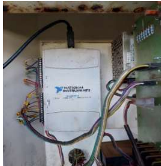
Data Acquisition Device
