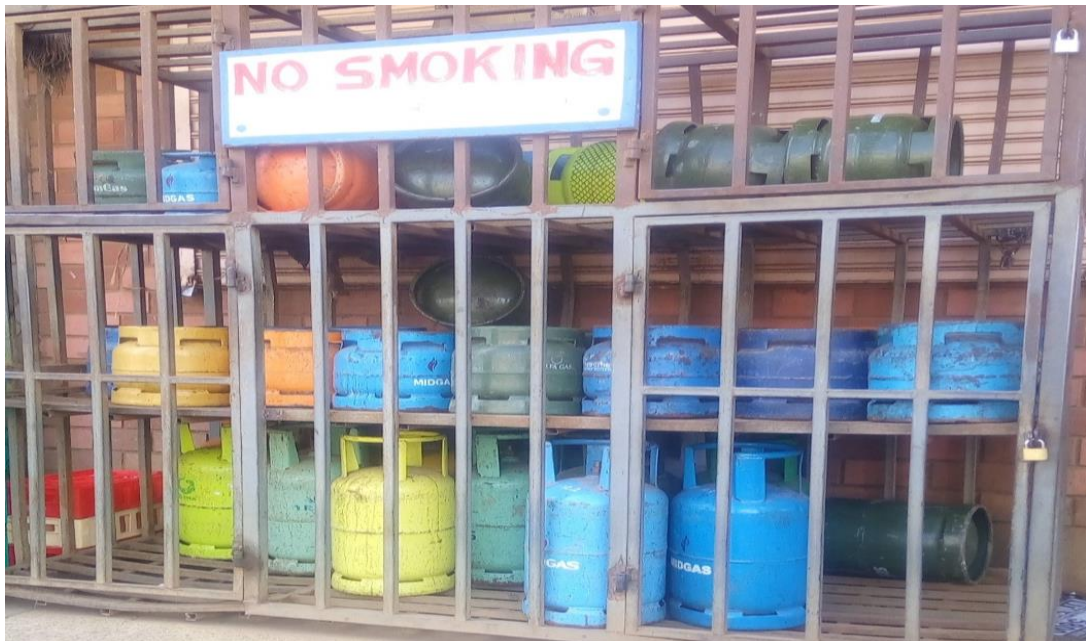
Bad practice: Poor cylinder storage (Cylinders stored horizontally, instead of upright position)
