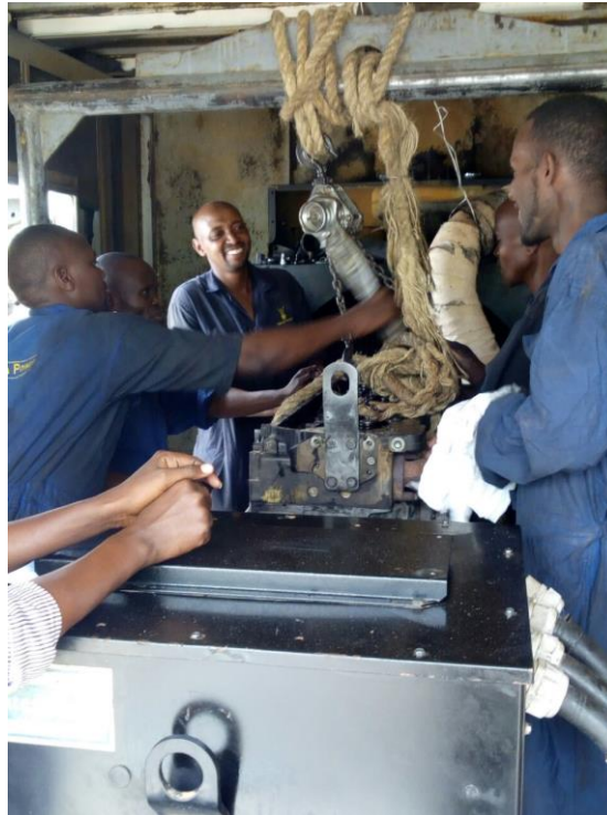
Figure 0.2 Kenya Power Personnel Repairing a Diesel Generator After Break-down 4
