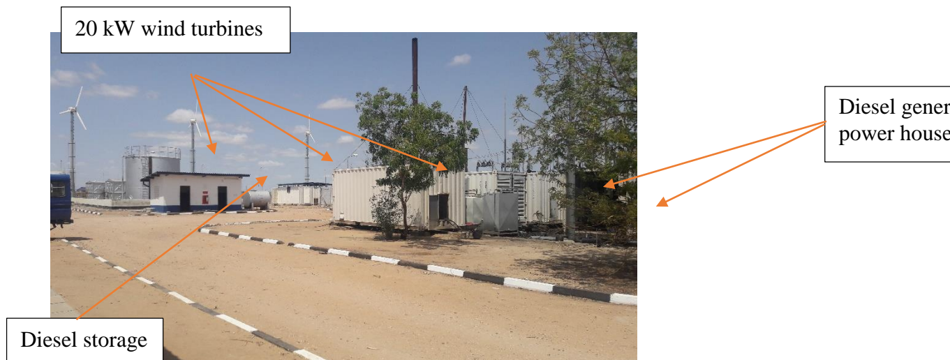
Figure 0.1 Photograph of Habaswein Power Generation Station
