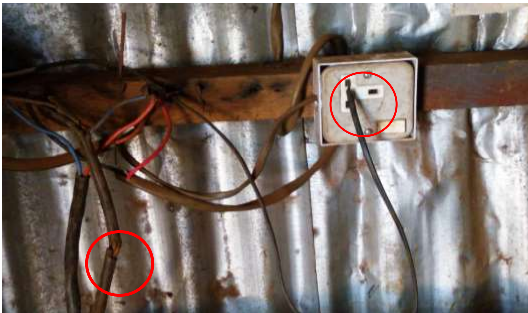
Photo 6: Naked electrical wires plugged directly into a socket without the use of a fused plug. Observed also are worn-out insulations on electrical cables, an electrical hazard.
