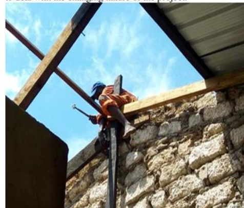
Plate 2: Roofer working without appropriate PPE
