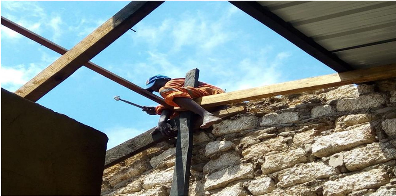
Plate 4.6 Roofer working without appropriate PPE
