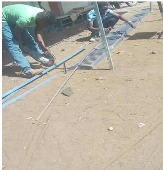
Plate 4.2 Workers in awkward posture and without PPE
