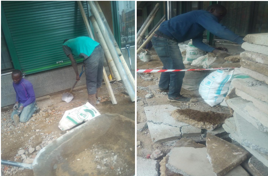
Plates 4.7 and Plate 4.8 Workers without PPE
