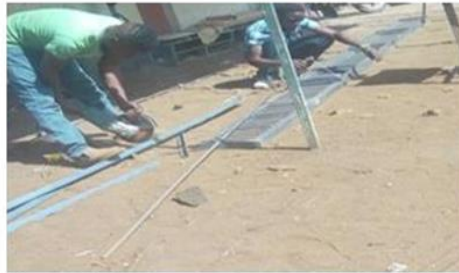
Plate 4.1 Workers in awkward posture and without PPE.
