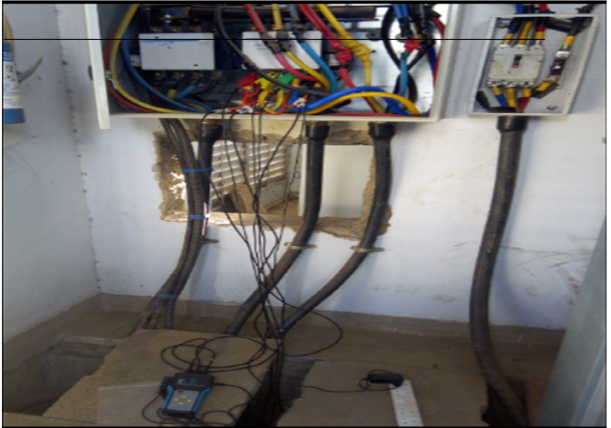
Figure 1b: ME 435 3-Phase Hand Hold Power Meter in Situ.
