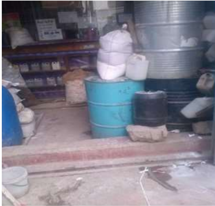
Plate 4.8: Normal route of entry obstructed with flammable and combustible material
