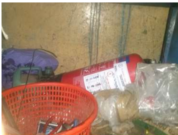
Plate 4.4: Wrongly placed fire extinguisher
