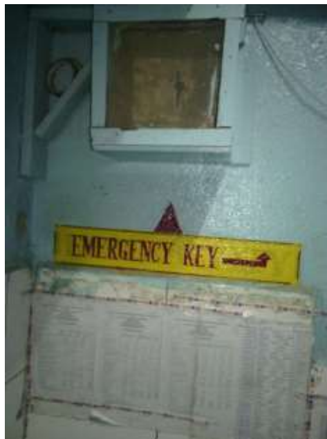
Plate 4.7: Emergency key box without a break glass hammer
