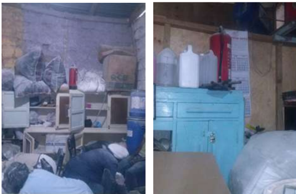
Plate 4.5: Fire extinguishers not mounted at the workplace
