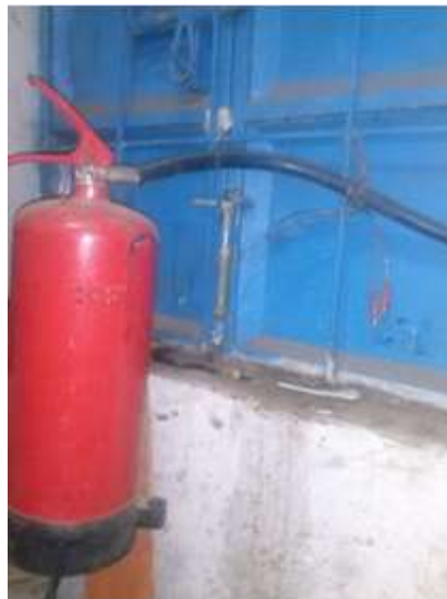
Plate 4.3: Fire extinguisher fastened by the discharge
