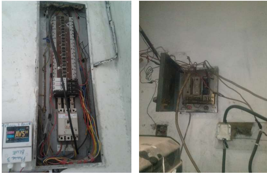
Plate 4.1: Exposed live electric wires
