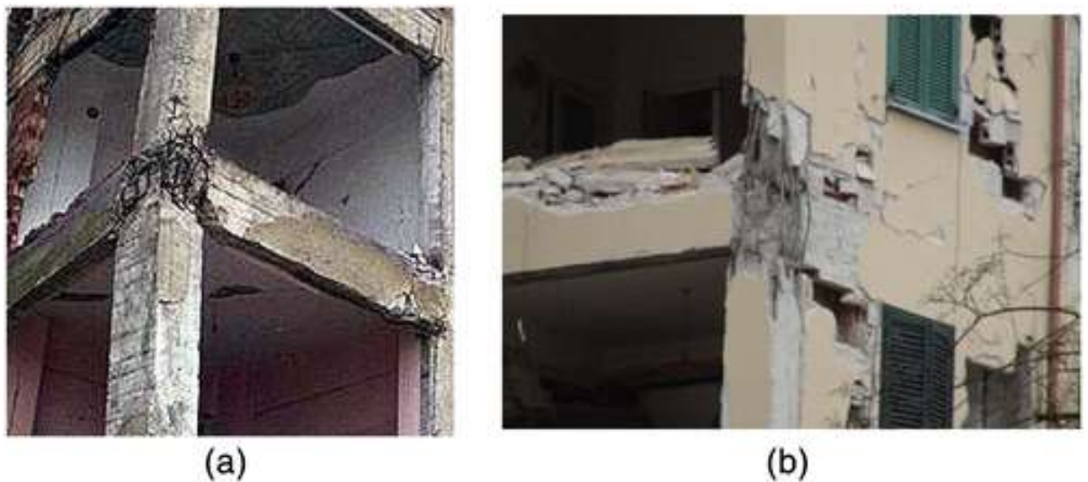
Figure 2- 5: Failure of corner beam-column joints in past earthquakes: (a) Izmit earthquake in Turkey 1999; (b) Abruzzo earthquake in Italy 2009
