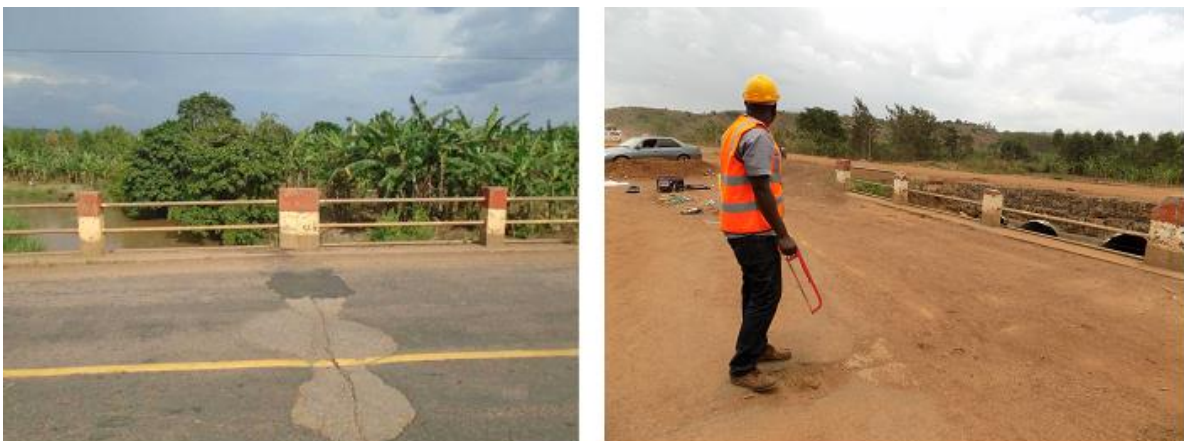
Plate 4-5 Transverse cracks in deck surfacing and concrete patching.
