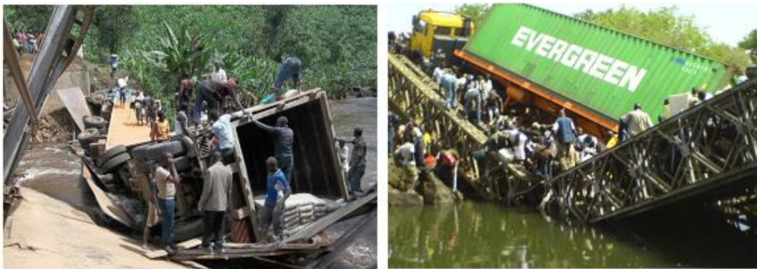
Plate 1-1 Collapse of the Mitooma Bridge and the Aswa Bridge respectively
