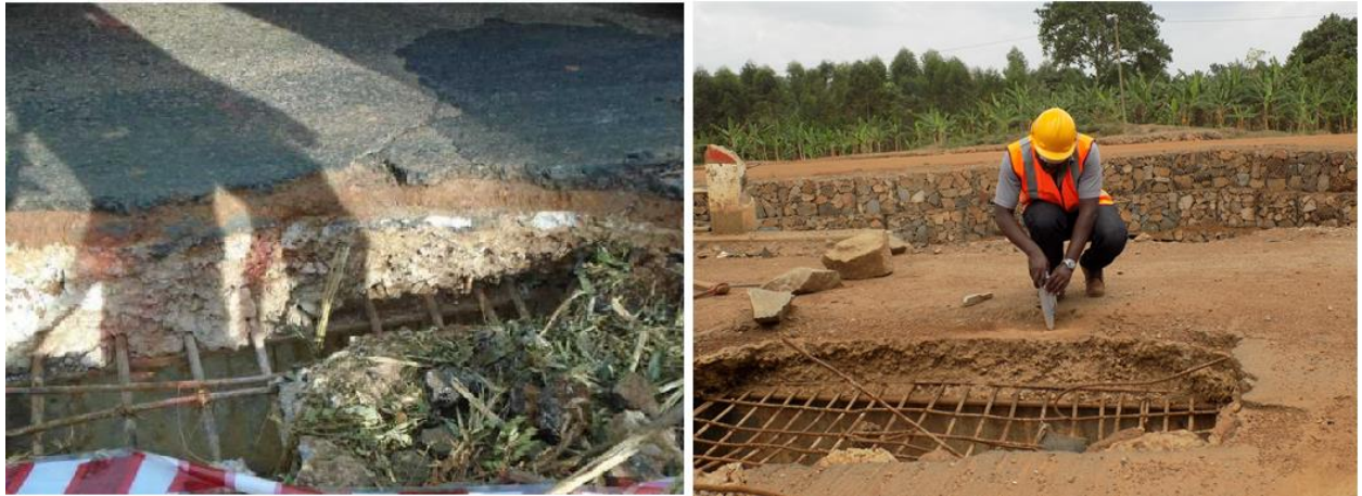
Plate 4-6 Opening in superstructure slab showing longitudinal steel beam, bottom reinforcement, disintegrated concrete layer and gravel layer under surfacing.
