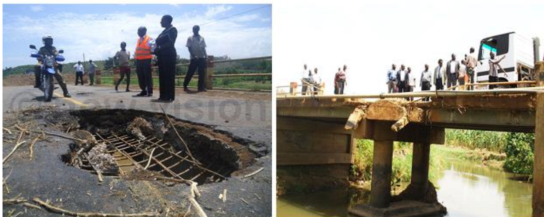
Plate 1-2 Failure of the Manafwa Historic bridge
