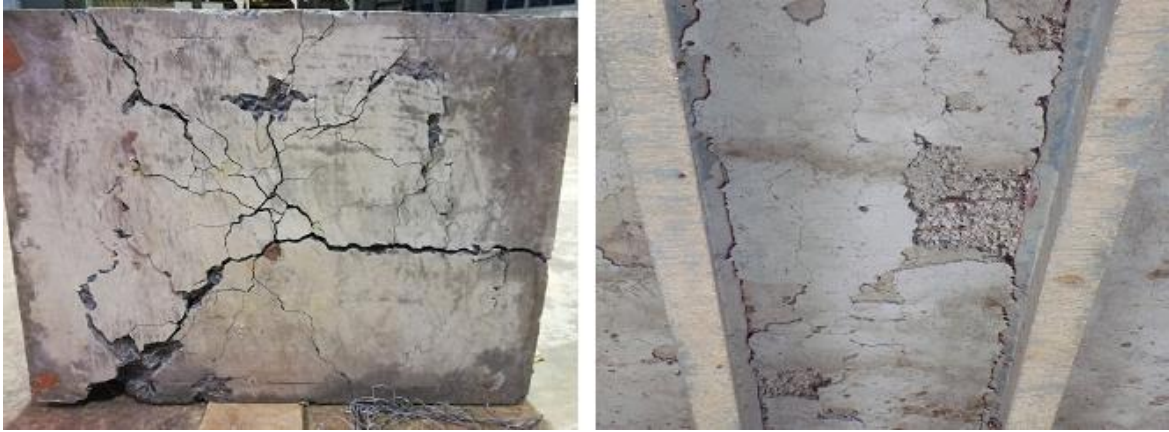
Plate 4-14 Bottom surface Failure of the Experimental model 13MPa deck slab vs Actual Bridge structure
