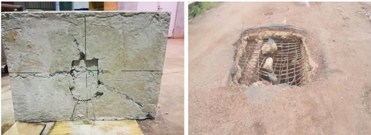
Plate 4-13 Failure in the Model compared to the actual failure in the bridge deck slab
