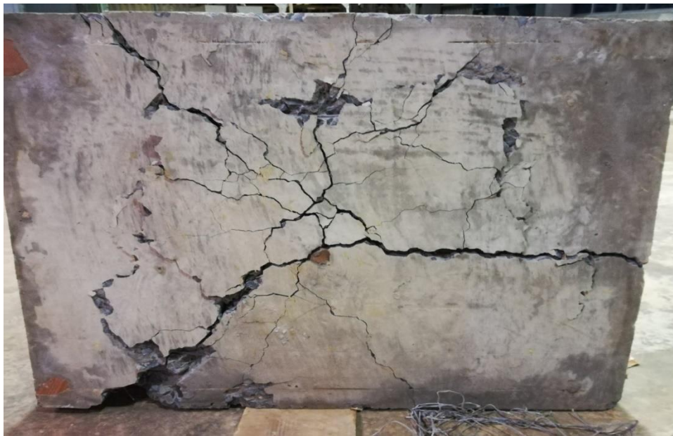
Plate 4-11 Failed Deck Slab – Indicates that the main cause of failure is punching shear regardless of the load but rather longitudinal cracking in the deck slab
