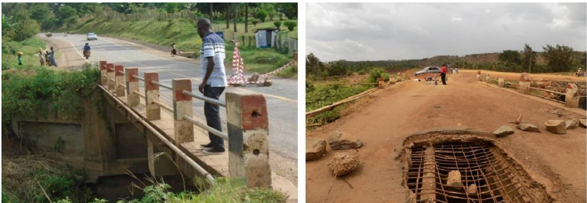
Plate 4-4 Manafwa River Bridge superstructure cross section immediately after the failure.
