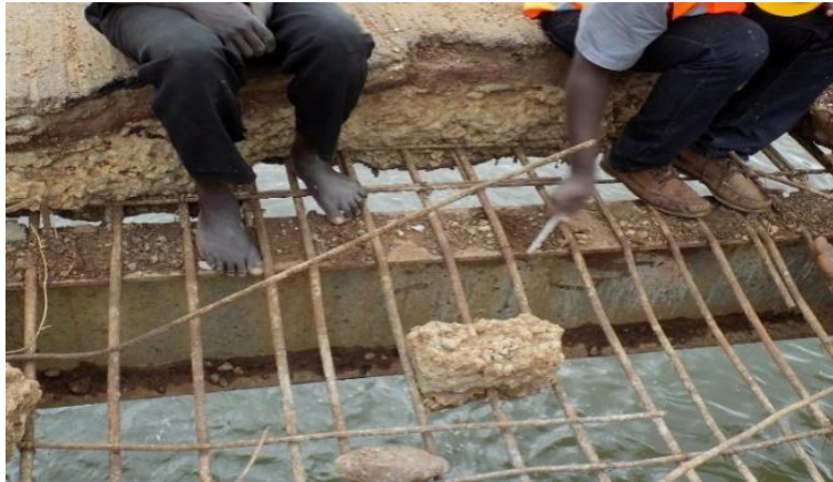
Plate 4-2 No hogging reinforcement in the slab, the concrete looks generally weak with a higher percentage of coarse materials
