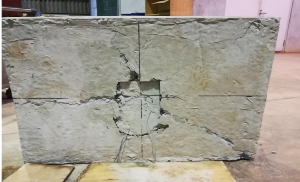
Plate 4-10 Total failure of the deck slab indicating that punching shear behaviour observed in the 13MPa deck slab was the main cause of failure for this model
