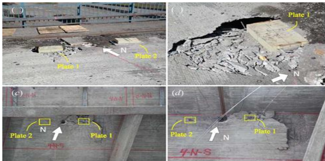
Figure 2-16 Failed bridge deck slab after shear failure
