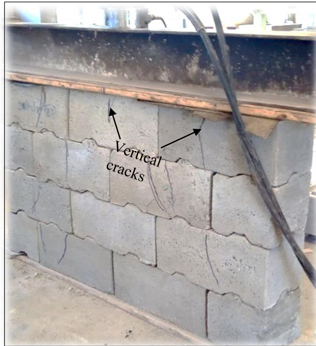
Plate 4.1: Vertical cracks parallel to the axis of loading for T-DHSBs wall model
