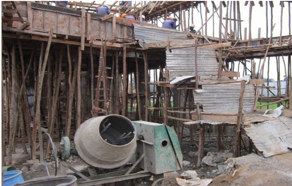
Figure 2.2: Platform prepared for placing concrete in the first floor of a building in Kenya Source: Field work, 2016.
