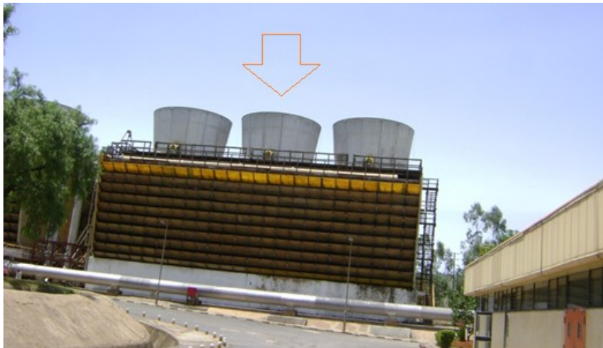
Plate 4.1: Cooling Towers in Olkaria 1 Geothermal Power Station
