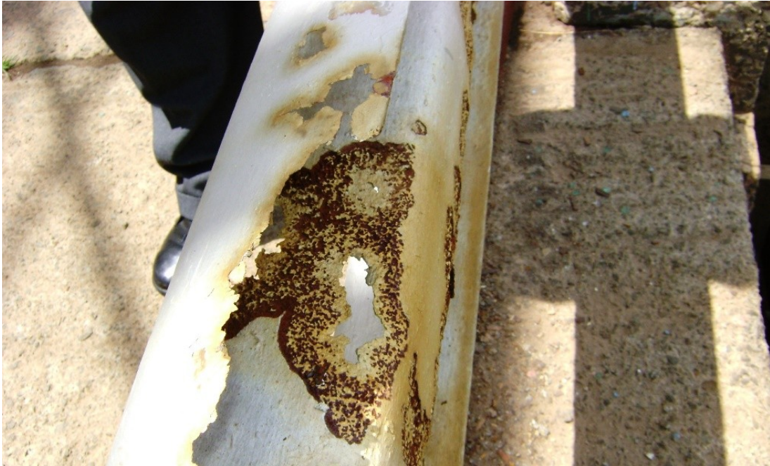
Plate 2.1: Corrosion of structures around seal pit in Olkaria I
