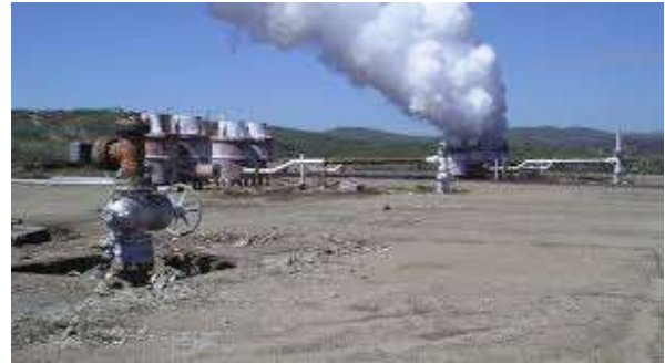
Geothermal plant at Olkaria
