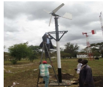
Installation of a 200W wind-turbine electricity generator at Saint Xavier Girls' Secondary School
