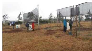
Fog harvesting equipment installed at Ilmasin Primary School in Ngong Hills,
