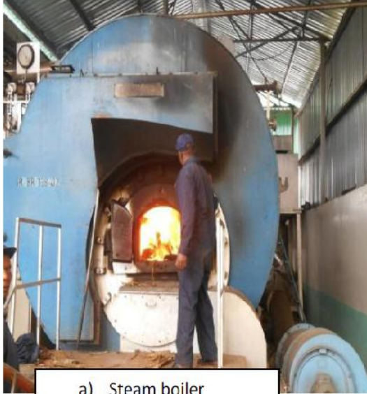
a) Steam boiler
