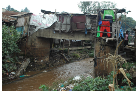
Plate 1.2.3: Informal trading encroaching on bridges. (Source: Author, 2007)
